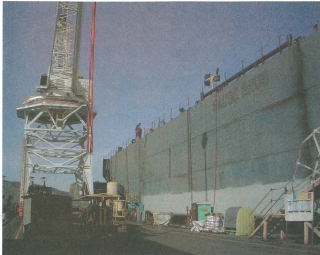
A Sause Bros. barge is shown here under construction at Gunderson's Marine facility in Portland
