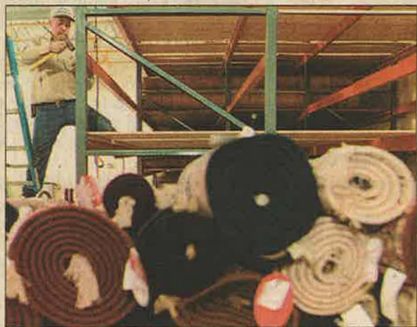
Ron Dees of R. Dees Construction finishes assembling racks that will hold hundreds of expensive rugs, some weighing 800 pounds each.
